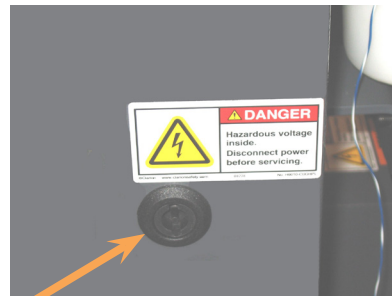
Special door lock.
