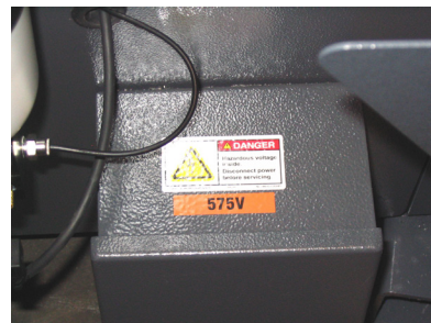
Power Junction Box.
